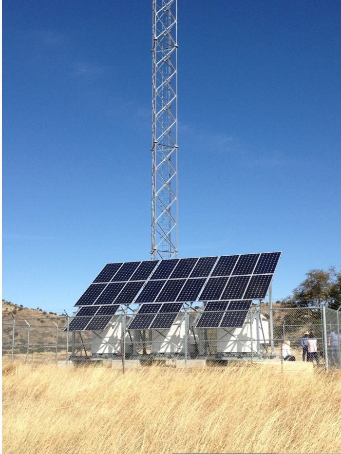
Large Cool Cell battery banks with integrated PV system. Monitoring Demonstration Project. Arizona Border
