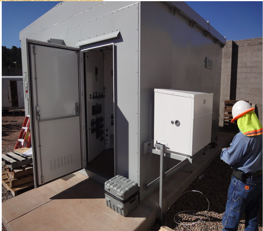
Locating the batteries outside creates more space inside and improves battery access. Zuzax substation, Zuzax, NM.
