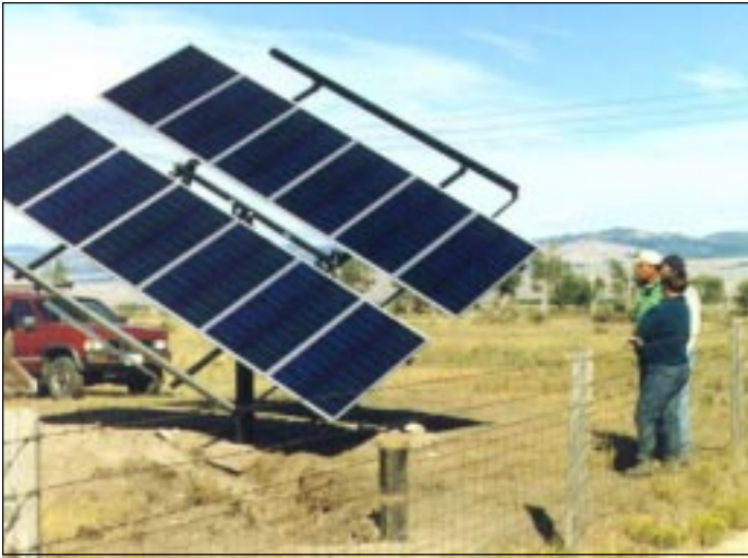
Solar pumping systems aren't just for summer use, as this project on Ueland Ranch near Anaconda demonstrates.
