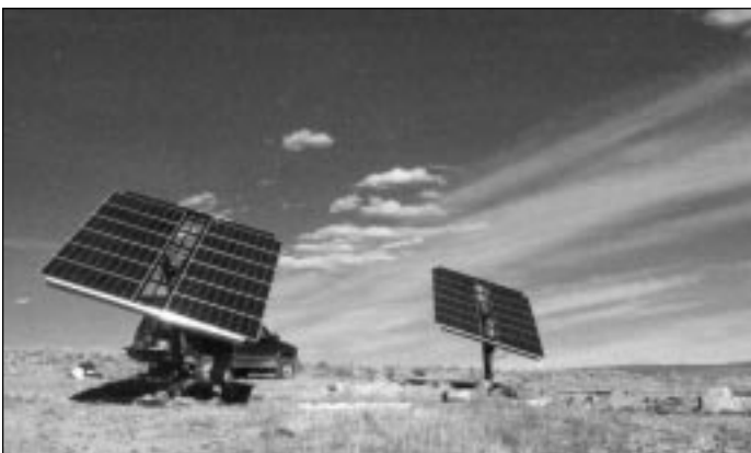
Twenty-four solar panels on the Sauerbier Ranch power a system that pushes water uphill to a storage tank over two miles away.
