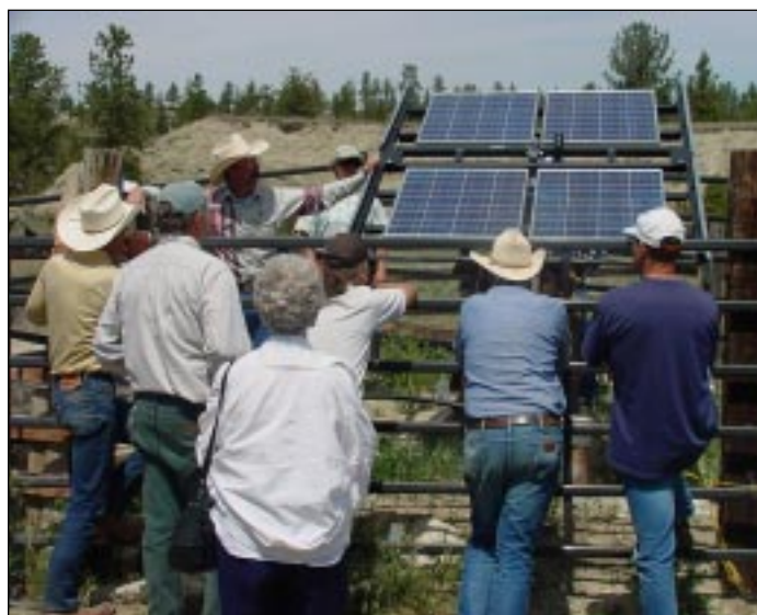
A tracking PV array replaced an old and unreliable windmill on the Ballard Ranch near Lavina.
