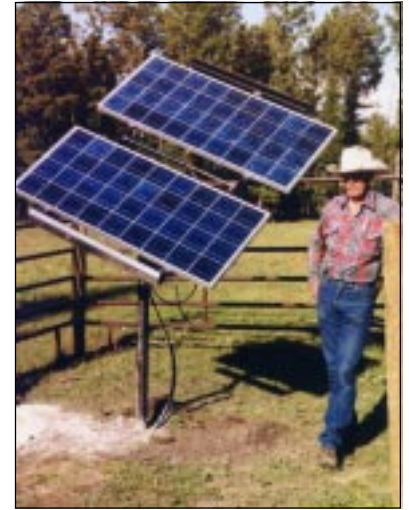
Solar pumping replaced a gas-powered generator on the Tomlinson Ranch near Gold Creek.
