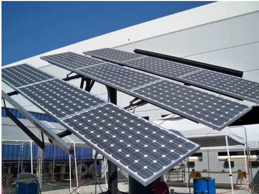
9 Panel Solar PV System for 3cu/m per hr flow rates
