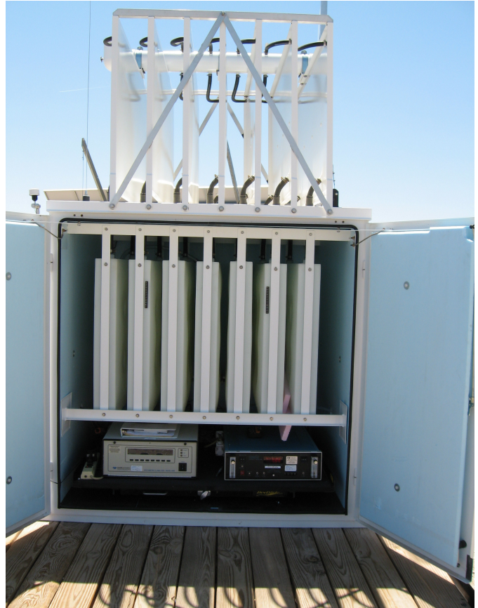
Trailer Mounted High Flux Cool Cell for Joshua Tree National Park Interior Showing Tanks, Radiators and Electronic Equipment
