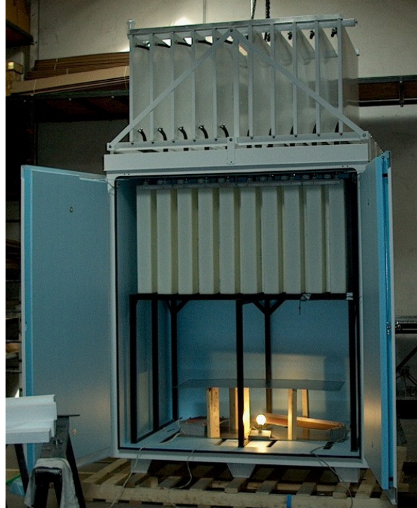
260 Watt High Flux Cool Cell Enclosure Test for ARAMCO Pipeline in Saudi Arabia. It Has 10 Radiators and 10 Tanks. These Have Been In The Field In Saudi Arabia For Three Years.
